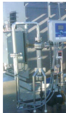
ILS used to remove solids from water supply system for a large grocery store.
